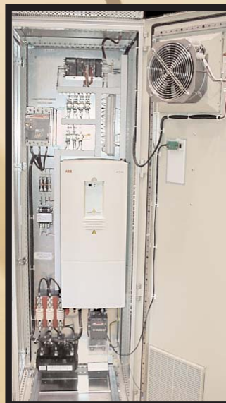
Press Drive Control Cabinet
